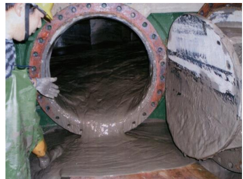
Photo 1 Mud Flow from Penstock Following Typhoon Aere
