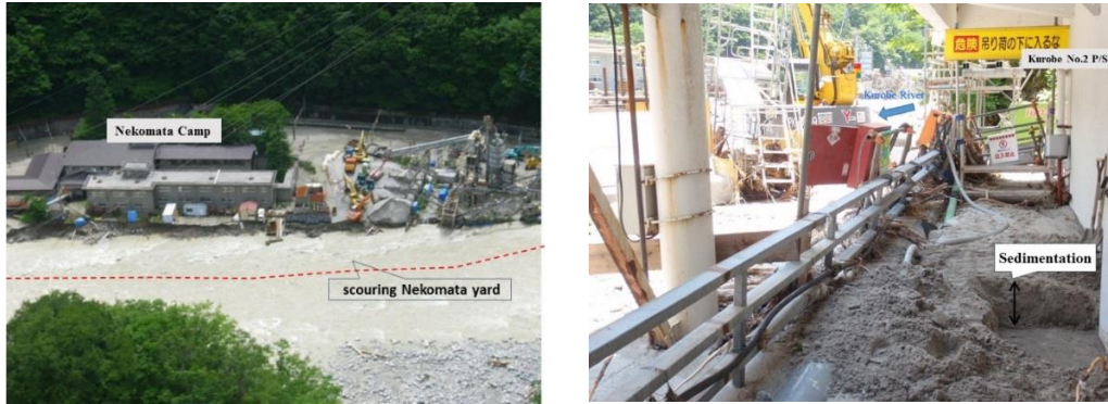
Fig.13 Damage by the flood in 2017
