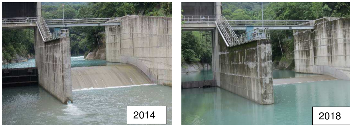
Figure 2: Sedimentation problem of Song-lin weir
