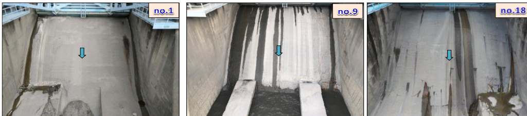
Wear pattern of the spillway
