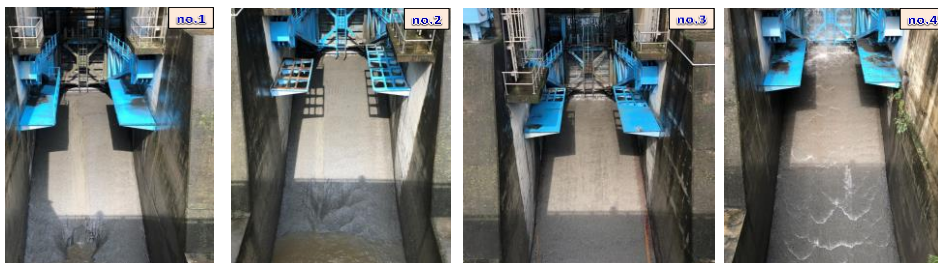
Wear pattern of the sluiceway
