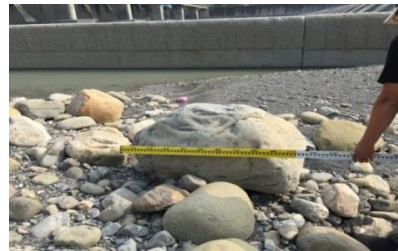
The rock staying in the stilling basin after flood.
