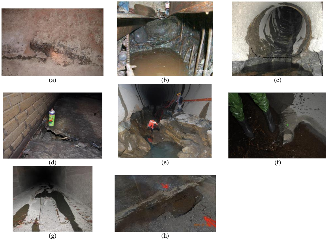
Figure 1: Case photos of invert abrasion in hydraulic tunnels: (a) Wushanling tunnel (Wang & Lee, 2013); (b) Mud Mountain tunnel (USACE, 2016); (c) Val d'Ambra tunnel (Hagmann, 2018); (d) Yuantanzi tunnel (UGI, 2013); (e) Palagnedra tunnel (Auel & Sumi, 2016); (f) Jiasian weir water delivery tunnel (UGI, 2012); (g) Asahi tunnel (Hagmann, 2018); (h) Yuanshantsu diversion tunnel (UGI, 2012).
