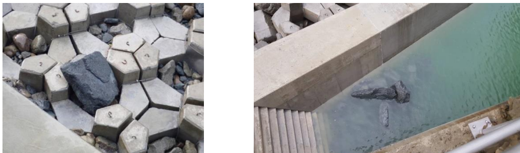
Figure 8: Photographs of concrete blocks in the outlet after trial run with water.
