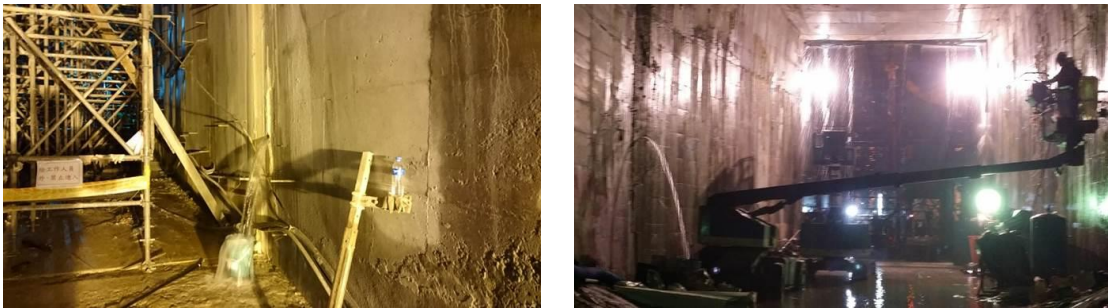
Figure 5: Water leakage of the lining during construction.
